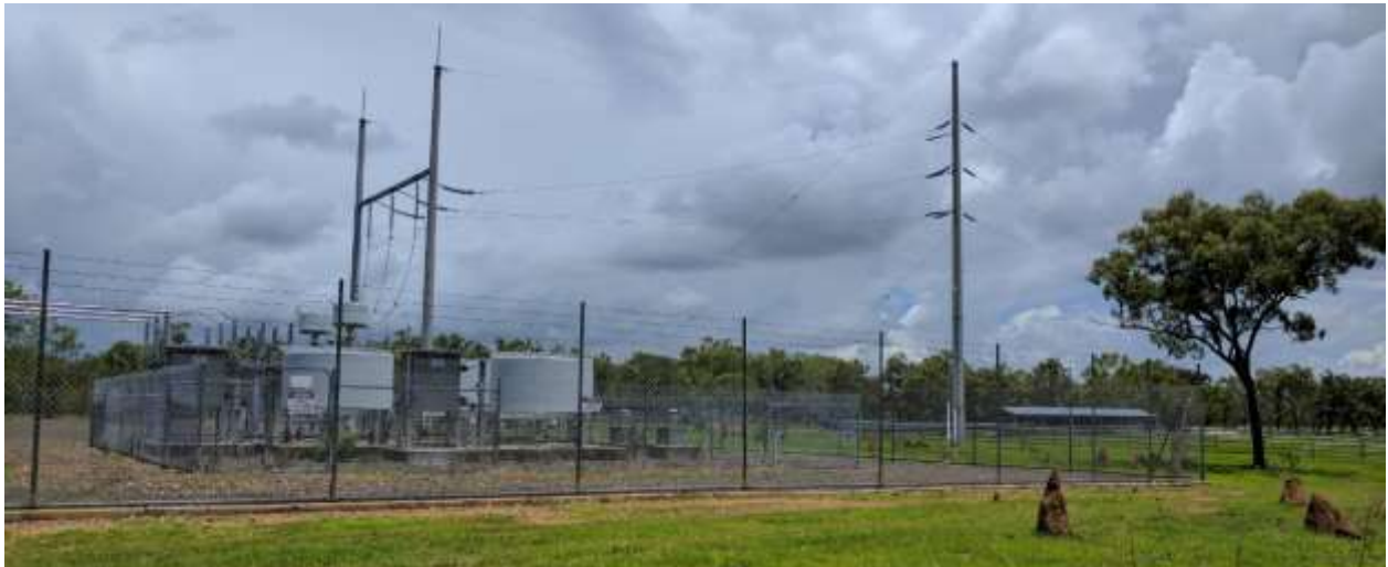
Lakeland Wind Farm will connect to Ergon Energy's electricity distribution network at their existing substation south of Lakeland
